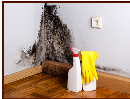
Moderate mold damage
