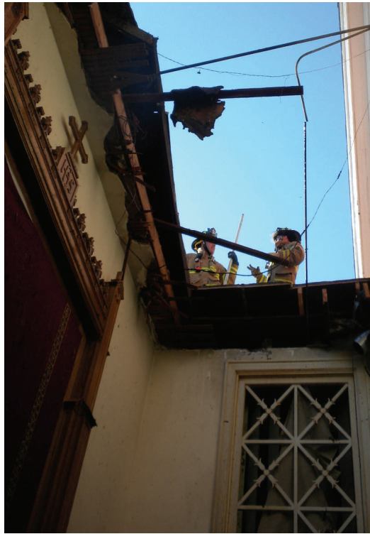
March 2010 church fire, electrical in nature.
